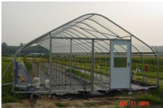
Figure 9. This high tunnel skeleton illustrates tall, vertical sides and peaked, or gothic, top and simple end walls that are desirable in high tunnel production.
