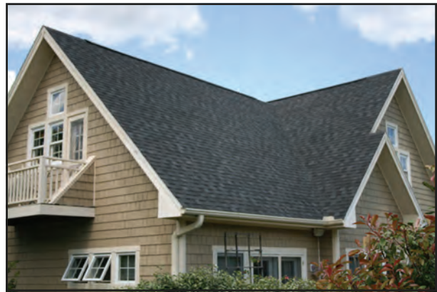
Figure 15. In the example above, about 25% of the total roof area feeds water to the downspout.
