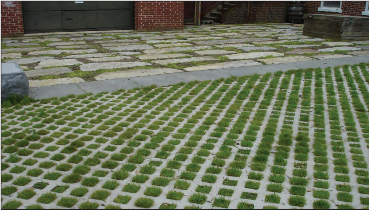
Figure 13. Permeable pavers installed at the Back Creek Nature Park in Annapolis, Maryland provide a solid ground surface that can support vehicles.
