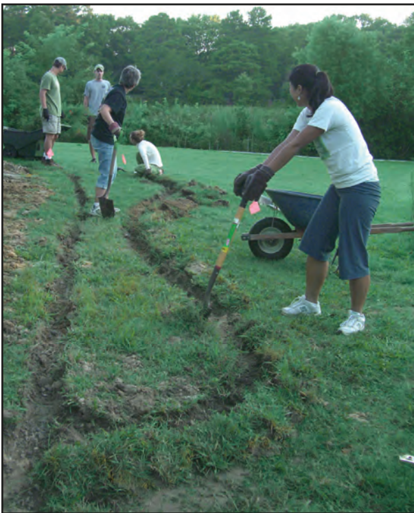
Figure 24. To construct the rain garden at the Ward Museum of Wildfowl Art in Salisbury, Maryland, the Lower Eastern Shore Tributary Strategy Team reused the garden area's sod to build a vegetated berm along the downslope side of the garden.
